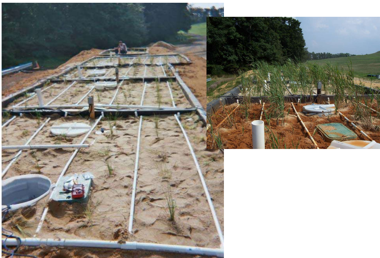
Figure 3: View of pilot WBS cells at Site A at completion (left) and after eight months of operation (insert right)
